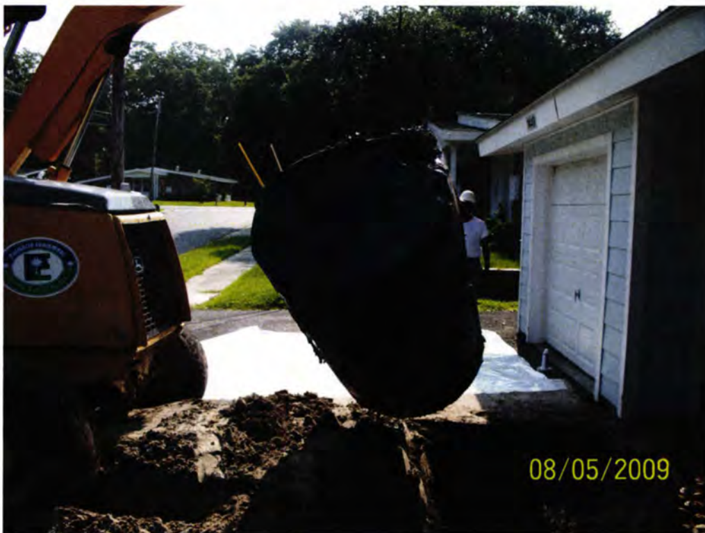
Picture 2: UST 1449Dove.
